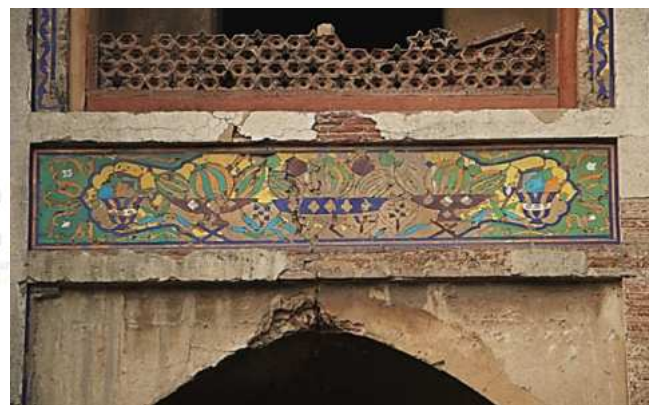
Fig. 9 Loss of Sandstone Jali Work
