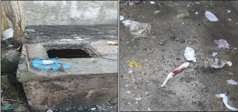
Figure 04 Operation theatre waste in an underground tank
