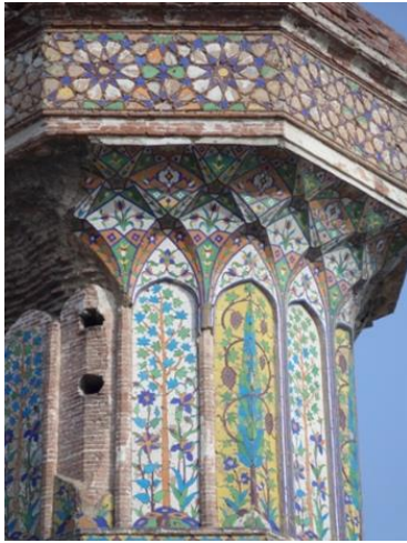
Fig. 15 Lost nMosaic Work and Dampness on base of turret
