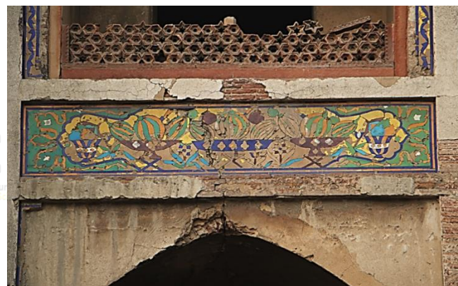
Fig. 9 Loss of Sandstone Jali Work
