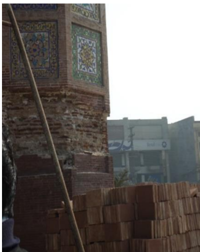
Fig.11 Lost Mosaic Work on Minaret
