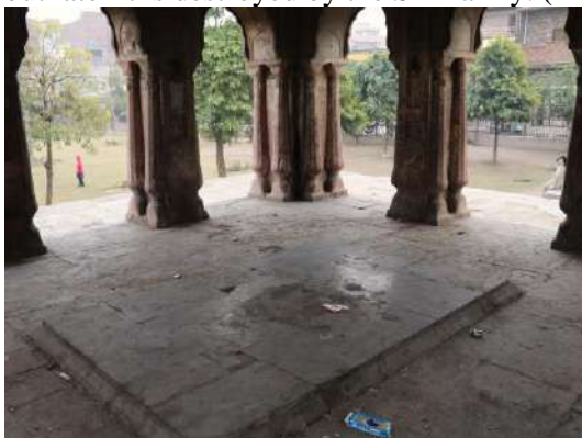
Plate.31 The podium inside the bārādārī , where the grave of Miān Nawāb Khān was constructed.
