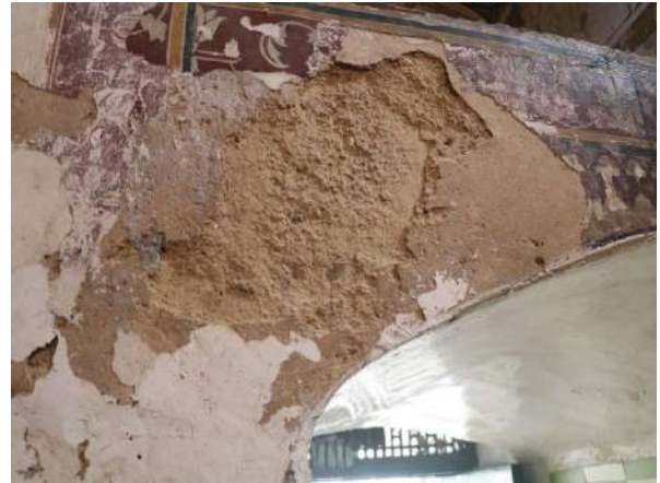
Plate.27 Damages of the beautiful structure of the tomb.
